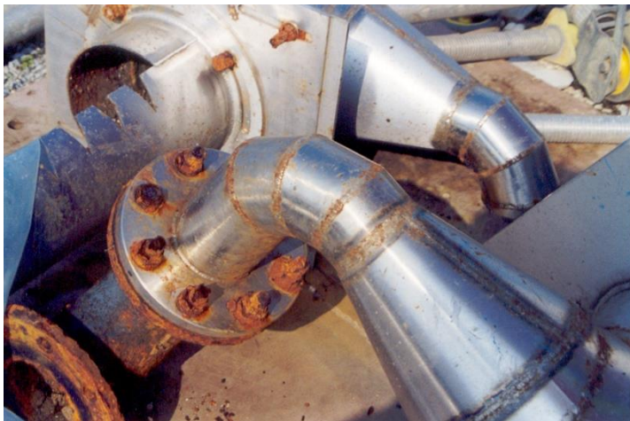
Figure 5-3 Heat tint and galvanic corrosion (© Roger Francis)
