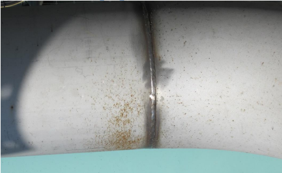
Figure 7-3 Corrosion of weld spatter (© Roger Francis)
